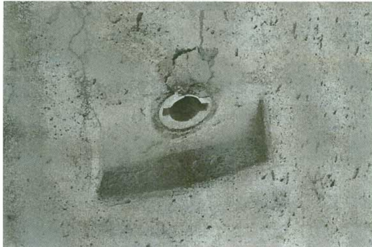
Spall and Damage Around Insert
