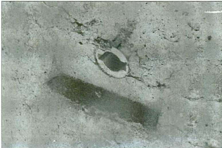
Voids and Poor Consolidation Around Insert
