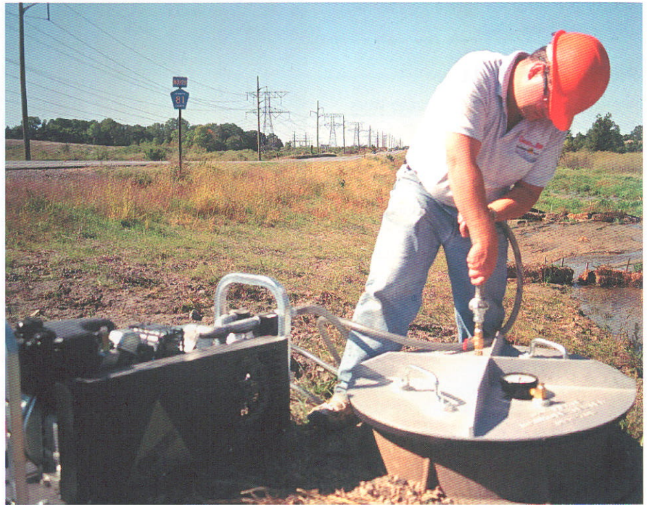
The use of vacuum testing is now the primary standard by which manholes are tested and accepted.
